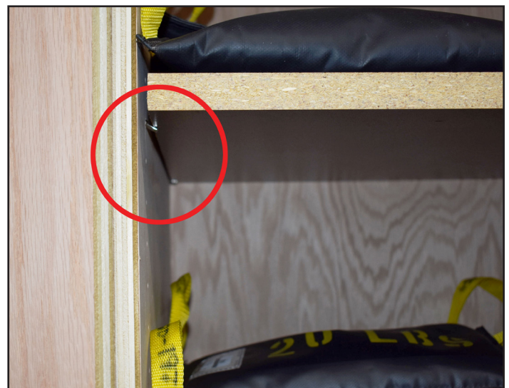
The above images illustrate the deflection of a single-pin shelf support system in veneer core tall cabinets loaded to the tolerances indicated on page 318 of the AWS Ed. 2 (2014) .
